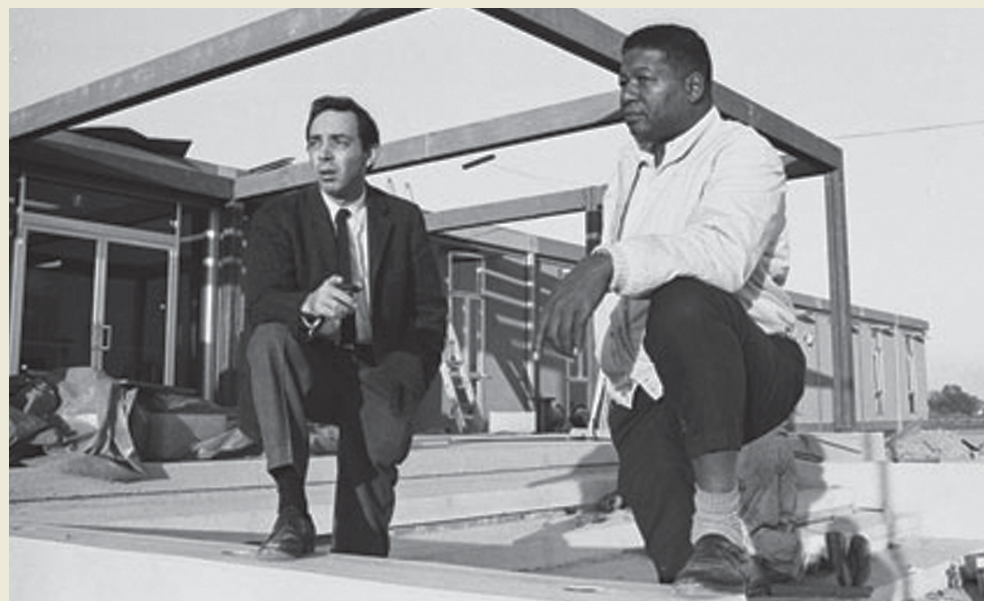
■ Dr. H. Jack Geiger and Dr. John W. Hatch during construction on the Delta Health Center, 1968.
